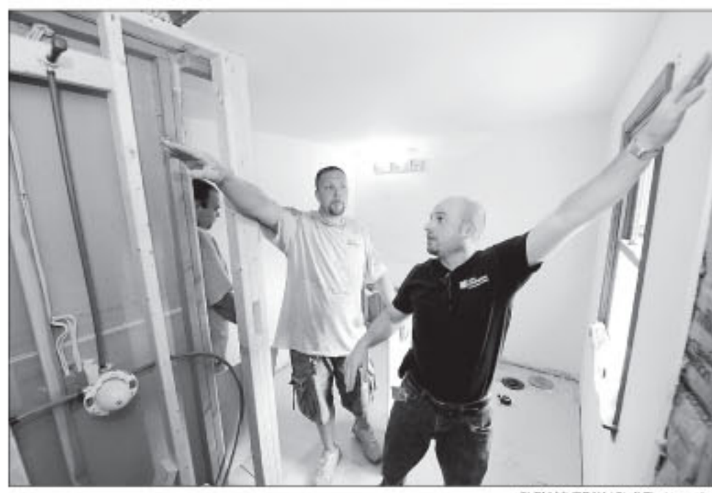
Bathroom Coordinator Adam Klein (right) of Anthony Home Improvements talks with contractor Paul Monteiro (left) about a bathroom-remodeling job they are doing in Chalfont. CLEM MURRAY / Staff Photographer
